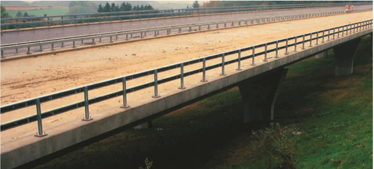
Figure 7.37 - A long viaduct on a slope as opposed to an embankment preserves the habitat and allows animals to move freely, as with this example of a Swiss motorway. (Photo by H. Bekker)
